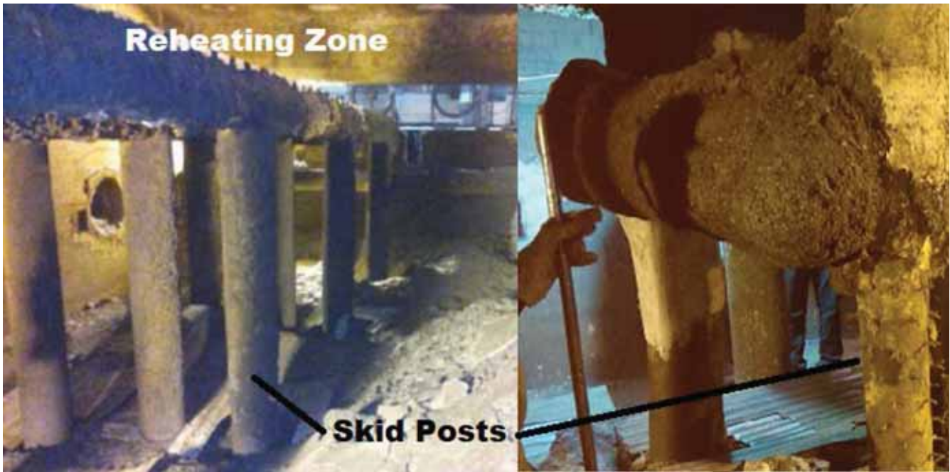
Fig. 1: Reheating furnace zone
